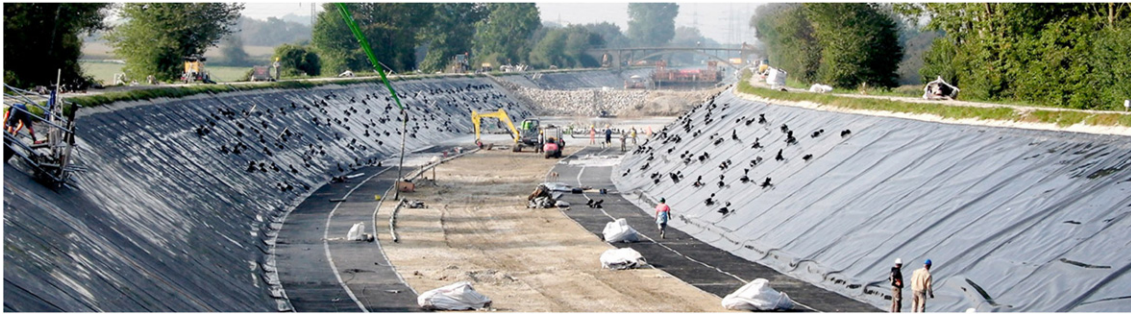
Figure 7. Use of a geomembrane as the lining in a canal (courtesy K. von Maubeuge Naue)
