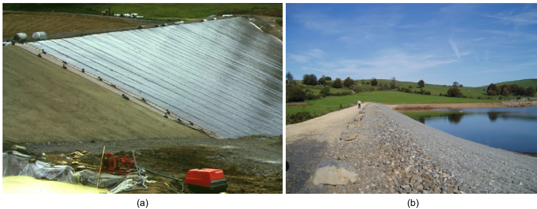
Figure 5. The Selvet dam (a) during geomembrane installation and (b) after completion and filling (courtesy D. Poulain)
