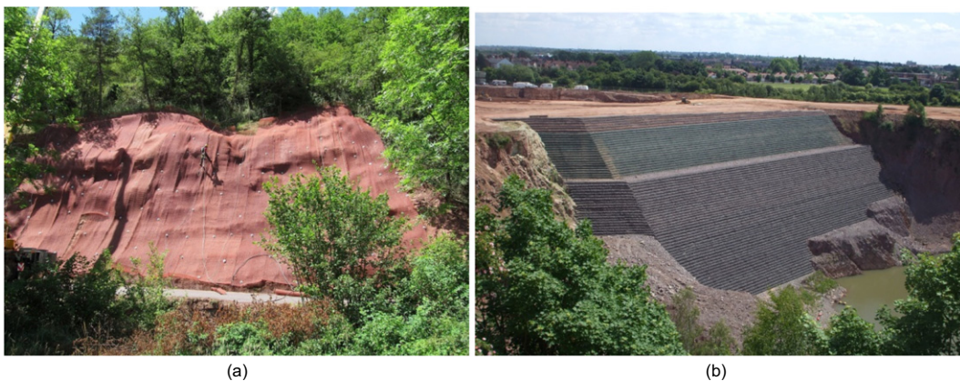
Figure 20. (a) Landslide prevention by using geosynthetics for erosion control. Winner French Chapter photo contest 2017 (courtesy Stéphane Pavlesk) and (b) Large reinforced soil structure just completed, IGS photo contest 2010 (P. Assinder)
