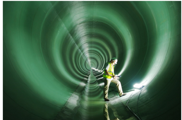
Figure 8. Use of a geomembrane in a tunnel, GIGSA photo contest 2015 (courtesy E. Zannoni)
