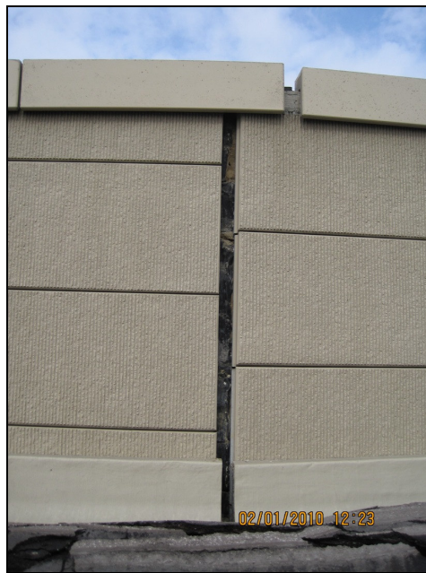
Figure 7 – MSE Wall Movement and Distress
