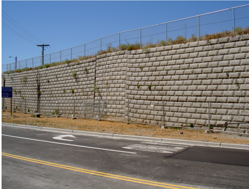
Figure 6 – MSE Wall Movement and Distress
