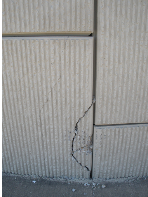
Figure 3 – Distressed MSE Wall
